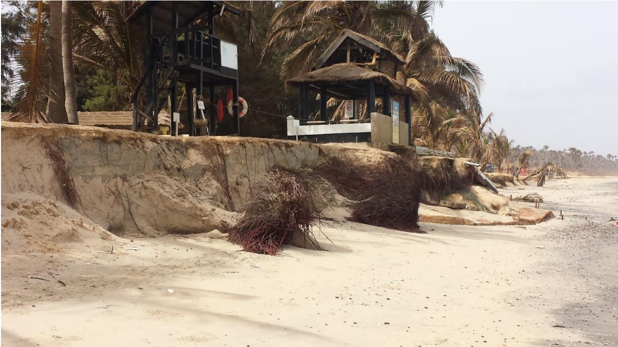
Figure 18: Frontage of the Kololi Beach Club; note the fallen coconut trees
