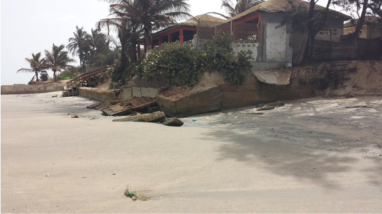
Figure 16: The Collapsed Frontage of the Holiday Beach Club Hotel
