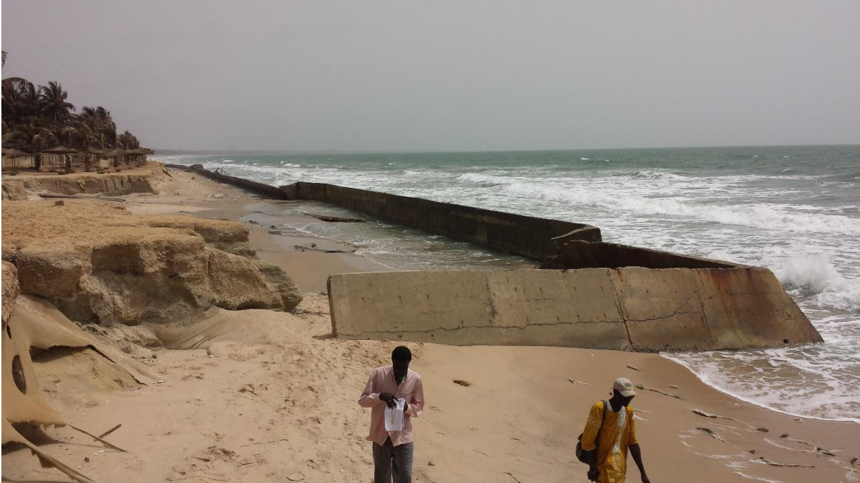
Figure 15: The Seawall at Kairaba Beach Hotel
